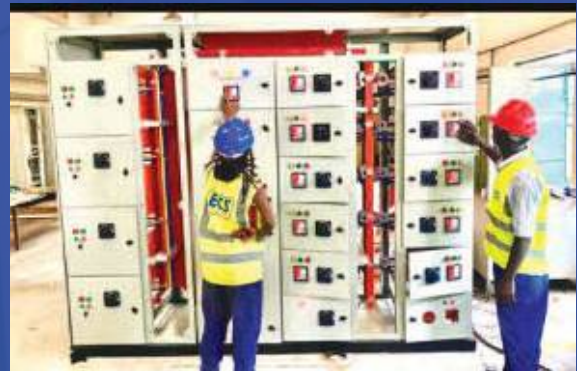
Power Distribution Board
