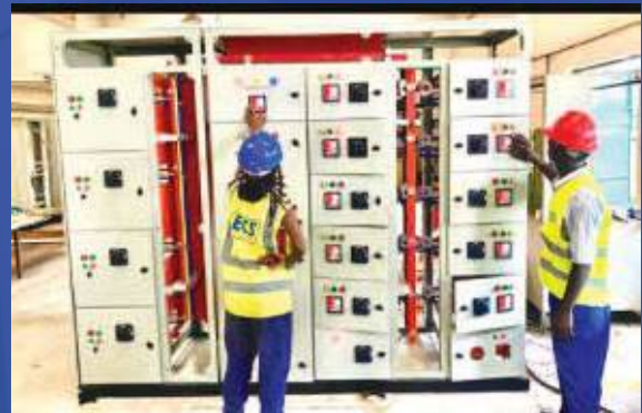
Power Distribution Board
